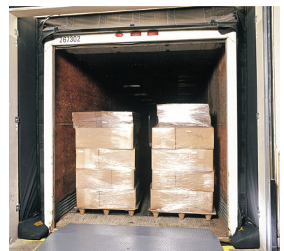
Ultra Dock Shelter – view from inside the warehouse
