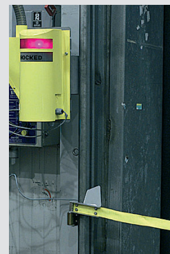
In positioned and showing red no go light
