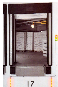
Dock Guidance Lights
